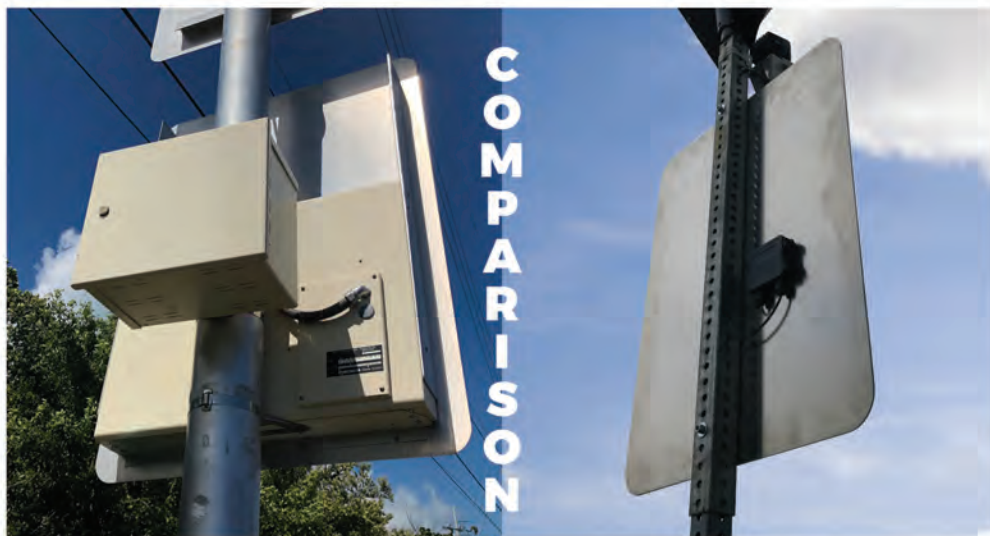
MOST COMMON LED SIGNAGE INSTALLATION
